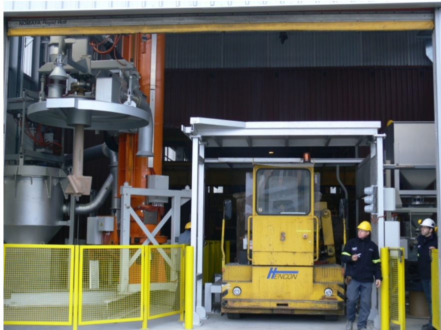
Figure 9. Metal treatment station.
